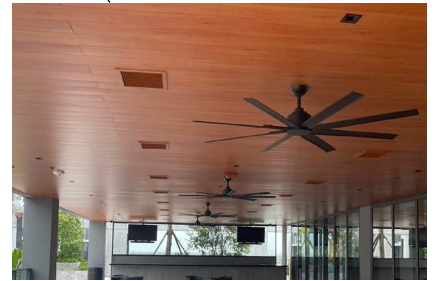
Conditioned Supply Air & Exterior Fans* *Power and Plenum provided by LL Fans, HVAC units and distribution furnished and installed by Tenant
